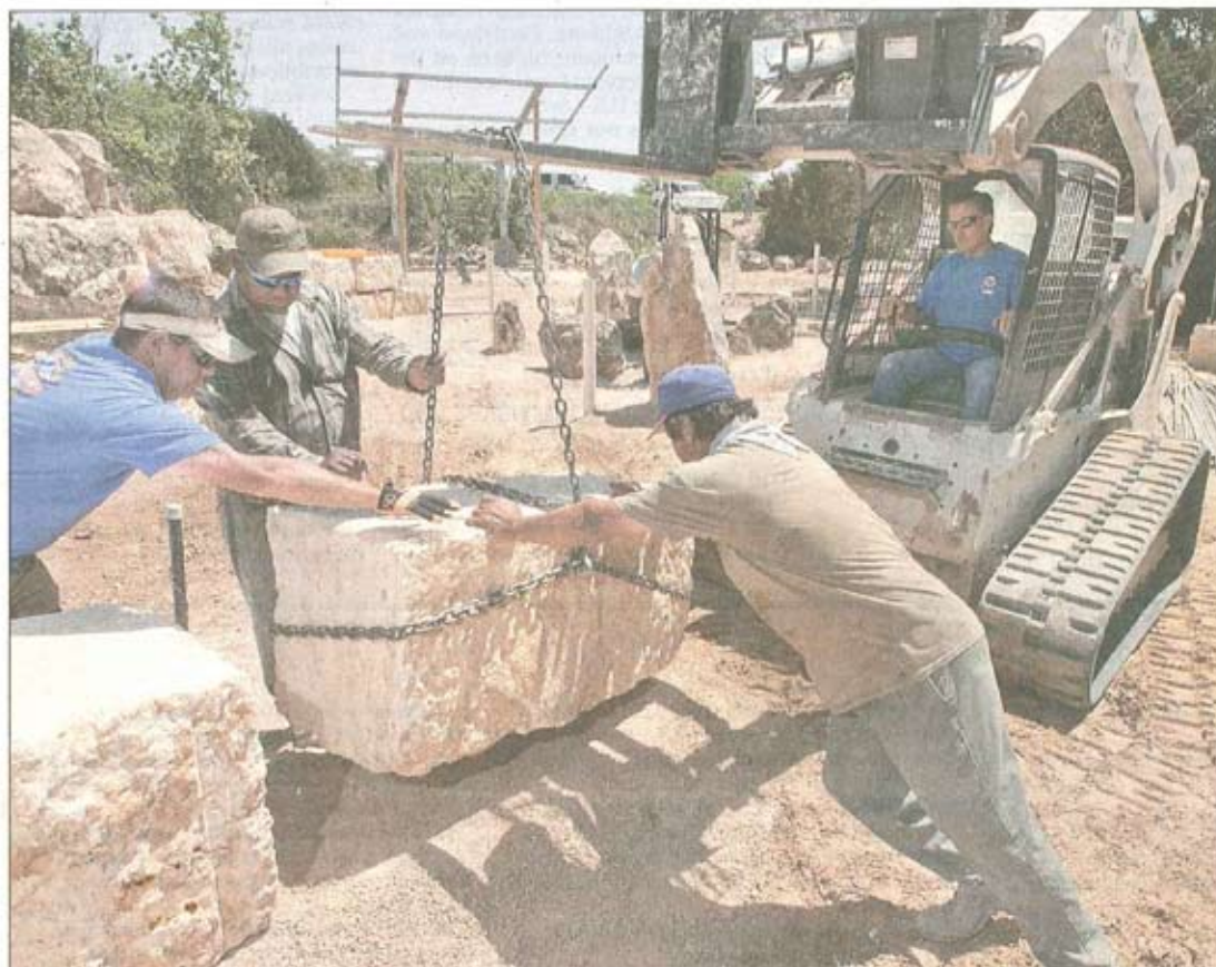
Workers move large chunks of limestone into place at what will become the Quarry Splash Pad, a water park at an old rock quarry in Williamson County. It is scheduled to open in mid-May. Williamson County is spending $1.8 million on this project, but the planned price of admission is a bargain: only $1 per person. See photos from the undeveloped rock quarry online at statesman.com/go/multimedia . Andy Sharp photos FOR AMERICAN-STATESMAN
